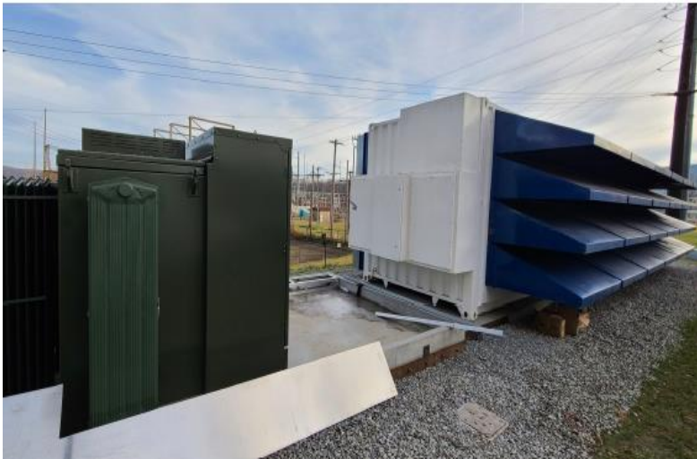
The Past (2017) – 2MW Self Contained Portable Data Center
