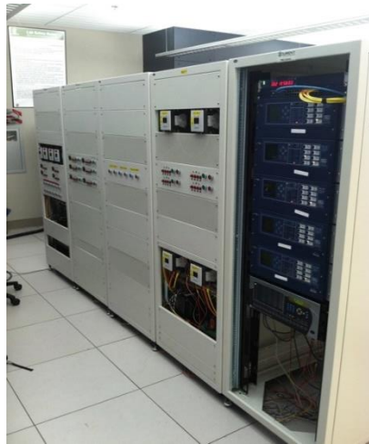
HTB Hardware room
