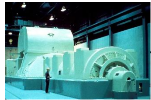
conventional generator or non-IBR ESS
